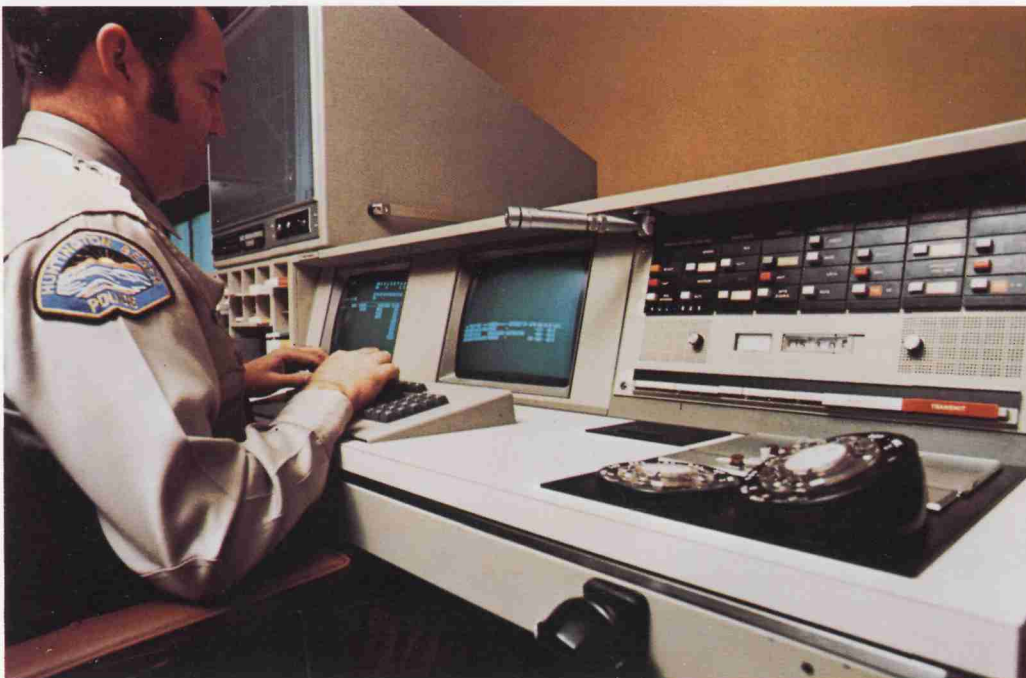
This Command and Control system, installed by Motorola in Huntington Beach, Calif., combines voice and data transmission to serve both police and fire departments.
